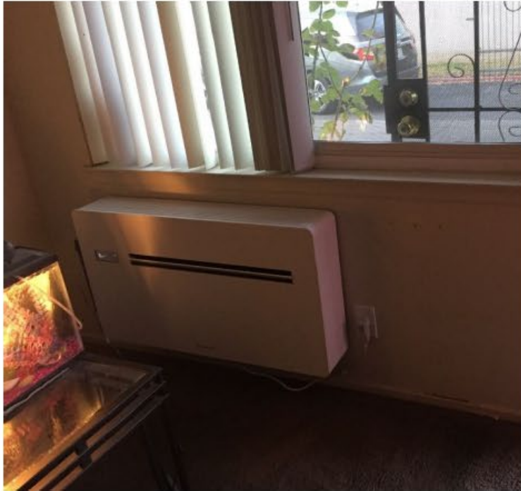
High Efficiency 120V heat pumps (140 units deployed)
