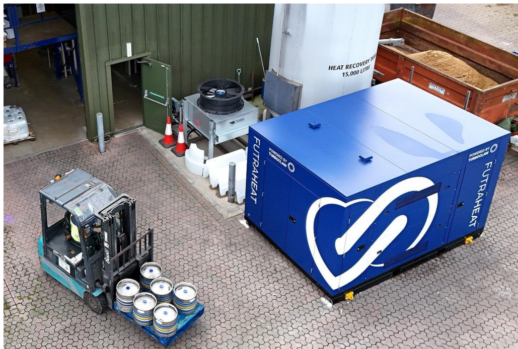
Figure 1: The Greensteam 330 installed at Hepworth Brewery
