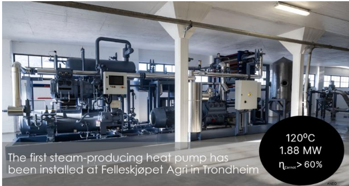
Figure 1: Ammonia heat pump and steam compression installation
