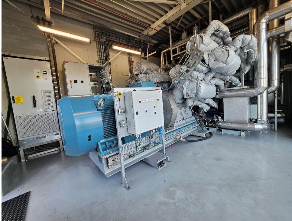
Figure 1: HighLift heat pumps currently installed Royal Friesland Campina, The Netherlands.
