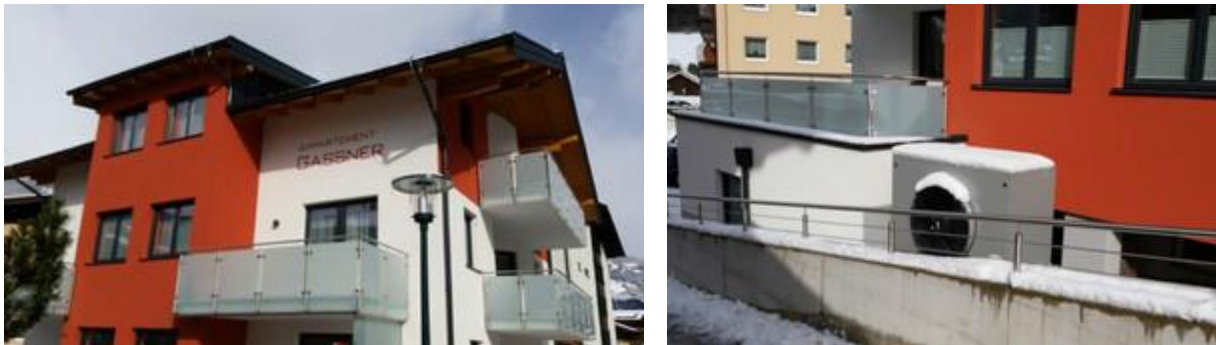
Figure 48: Pictures of the system in Bad Hofgastein (Glen Dimplex Deutschland GmbH, 2017)
