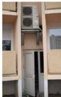
HP outside unit
