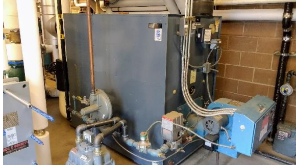
FIGURE 8 - TWO HHW PUMPS
