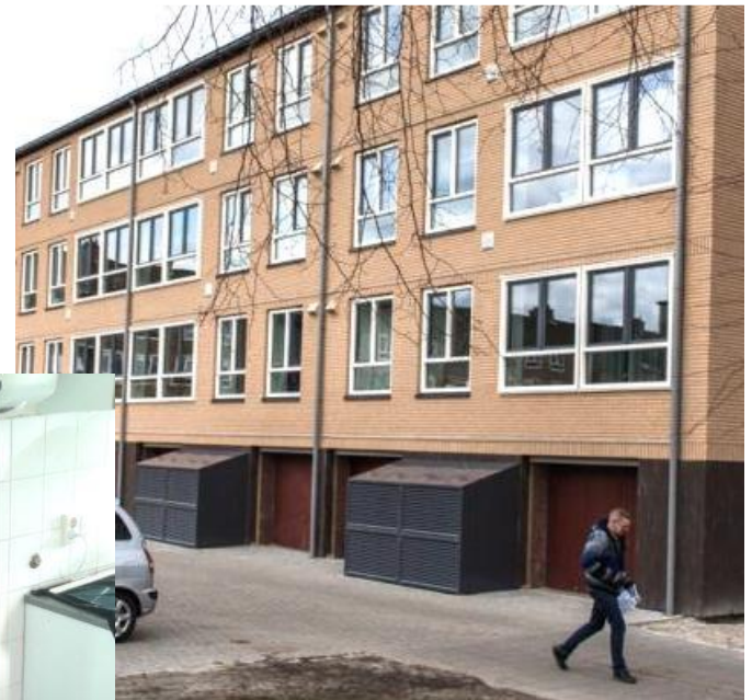
Casings at the entrances to accommodate three Mitsubishi air source evaporators.
