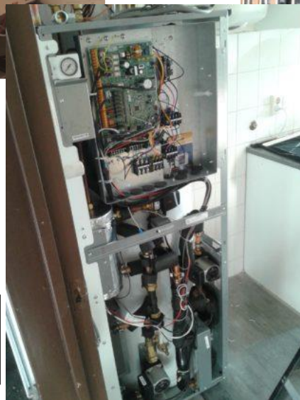
In the project, an individual heat pump was chosen, of which the indoor unit will replace the old gas boiler.
