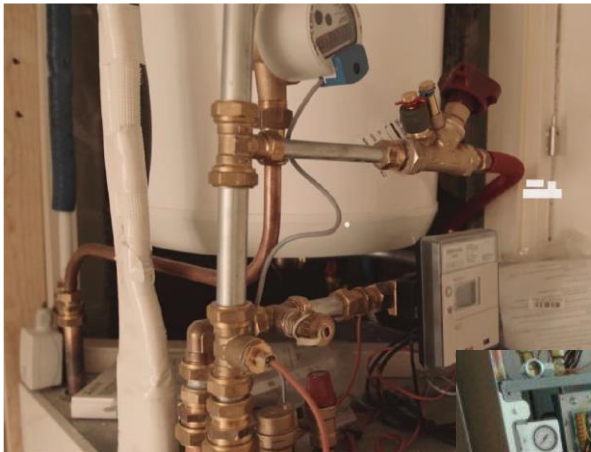
Hot water storage tank (100 litres) with smart metering inside storage cabinet in each apartment
