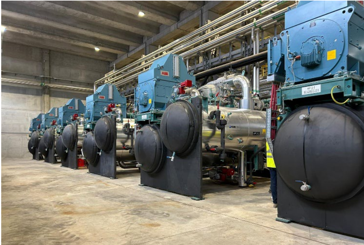
Figure 3: The Brescia (Italy) waste-to-energy plant is one of the largest in Italy. In the picture are represented 6 (of the total 9) Large Heat Pumps to recover the heat from the flue gases of the waste-to-energy plant, with a total heat recovery capacity of 60 MW.
