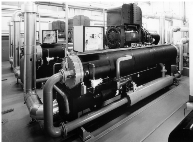
Large heat pumps (4.5 MW) use waste heat from river water power plant and supply district heating system, Birsfelden, 1984
