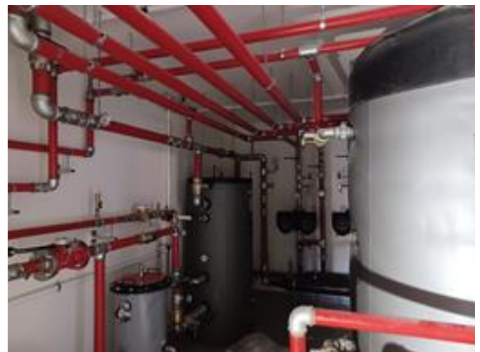
Installed heat pumps: Edge EVO 14.1 (31,8kW each)
