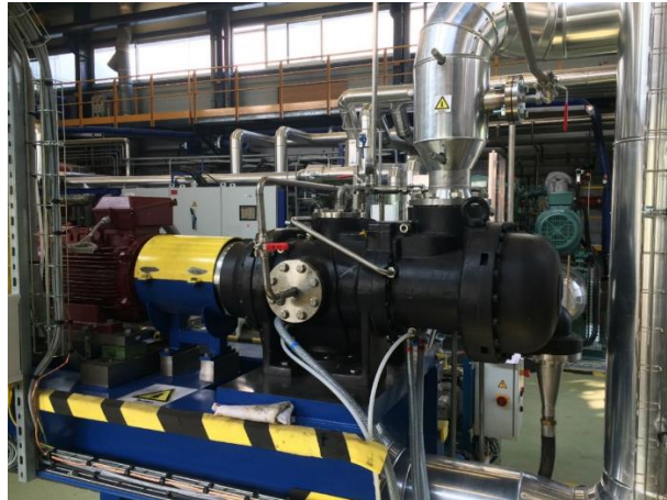
Figure 2-18: SRM prototype compressor skid.
