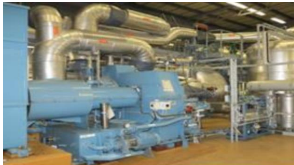
Figure 4-19 An existing Siemens energy heat pump 4
