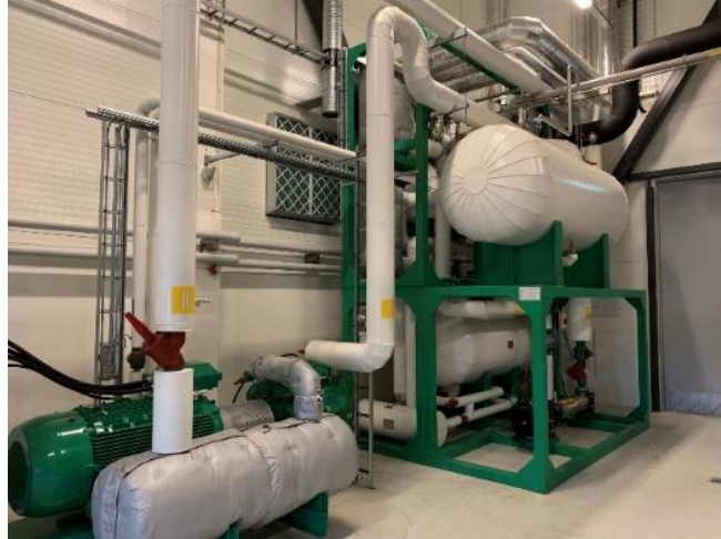
Figure 2-24: GreenPAC heat pump from Hybrid Energy at TINE Bergen.
