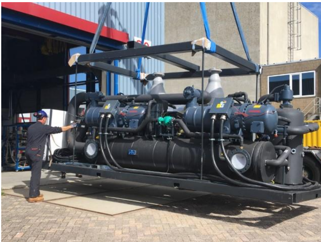
Figure 4-42: LowCapEx heat pump being installed at TNO testing facilities.
