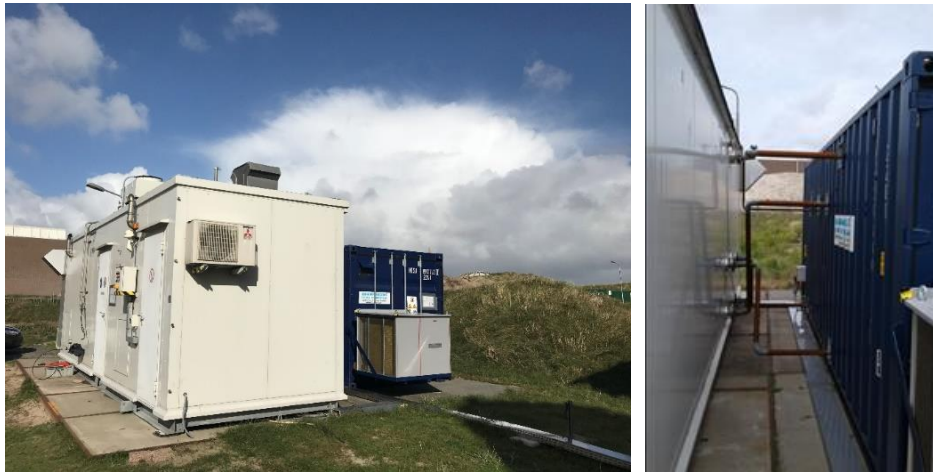
Figure 4-41: Heat pump (left) coupled to specially designed test rig (right).
