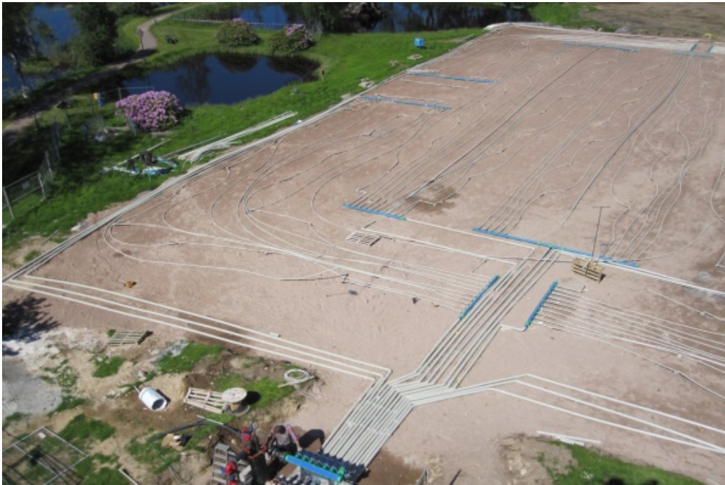
Figure 6: Photo from the summer 2010 showing the horizontal pipe system (gray) on top on sand. The blue colored pipes on the surface are field manifolds and in mid bottom one out of two main manifolds, now placed in the storage technical room. (Photo: Leif Rydell)
