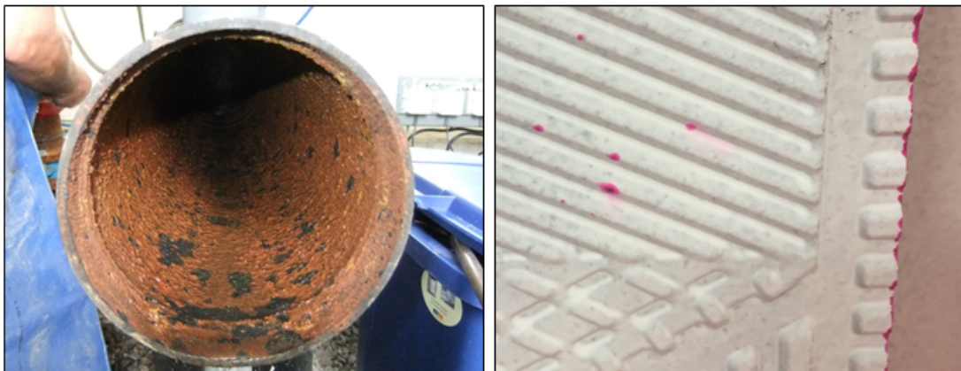
Figure 28: Left, general corrosion inside the culvert. Right, pitting corrosion on a heat exchanger plate (pink color)
